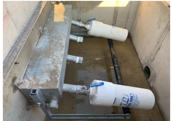
SKID 1x4 PETRO PIPE concrete inspection chamber connected to a transformer retention pit - EDF
