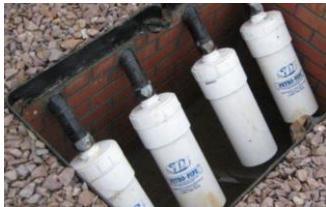
PETRO PIPE PI-616-M2 filters mounted in parallel
