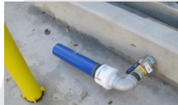
PETRO PIT 416 filter installed on a concrete retention basin
