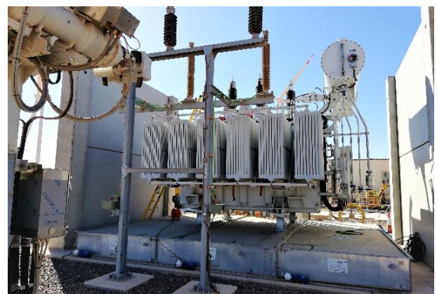
TRT-MODULO 3 Tank equipped with an EXTICOV LHD fire-resistant cover and PETRO PIT SPI filtration cartridge - DALKIA
